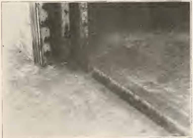
Even with the completely ratproofed buildings, sliding doors flashed with metal and fitting snugly in the groove of the concrete floor are necessary to keep the rats from coming in and out.
